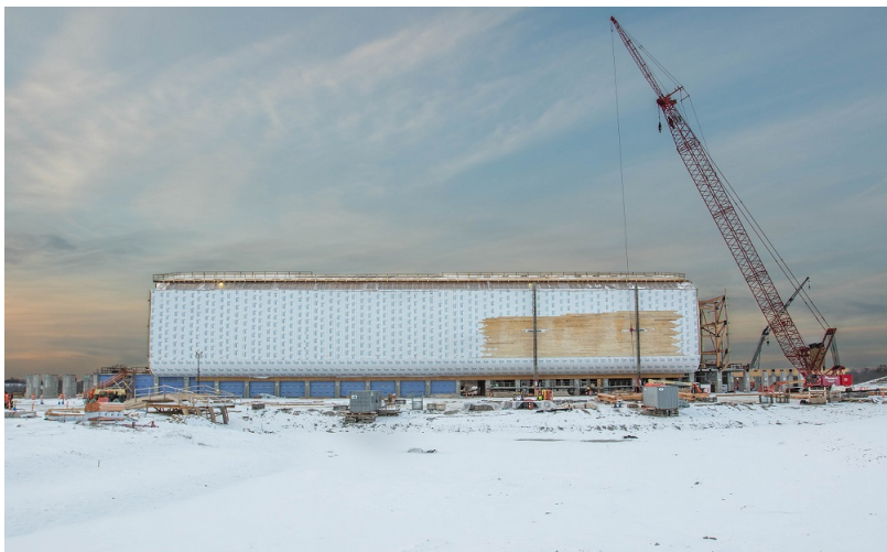
A wide shot of the Ark Encounter in the snow. The skin is being applied as the keel is being built out. Photo taken January, 2016, provided courtesy of Answers in Genesis.
